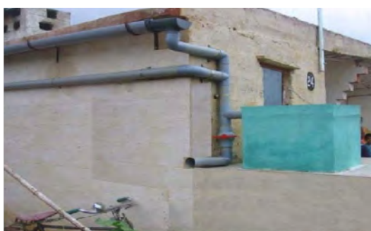
Fig. 3.47 Roof top rain water harvesting
