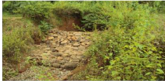
Fig. 3.28 Gully plugging Source: Authors' own collection
